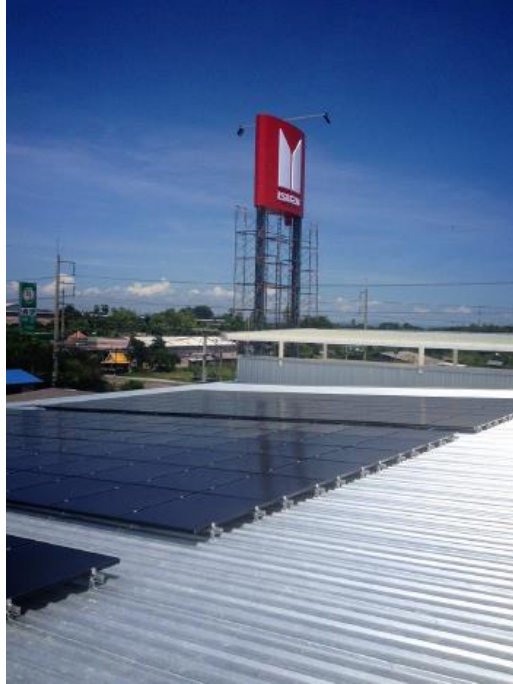
50kW CIS rooftop system on Isuzu car dealership in Ratchaburi, Thailand (Photo courtesy of Energy Pro Corporation)
