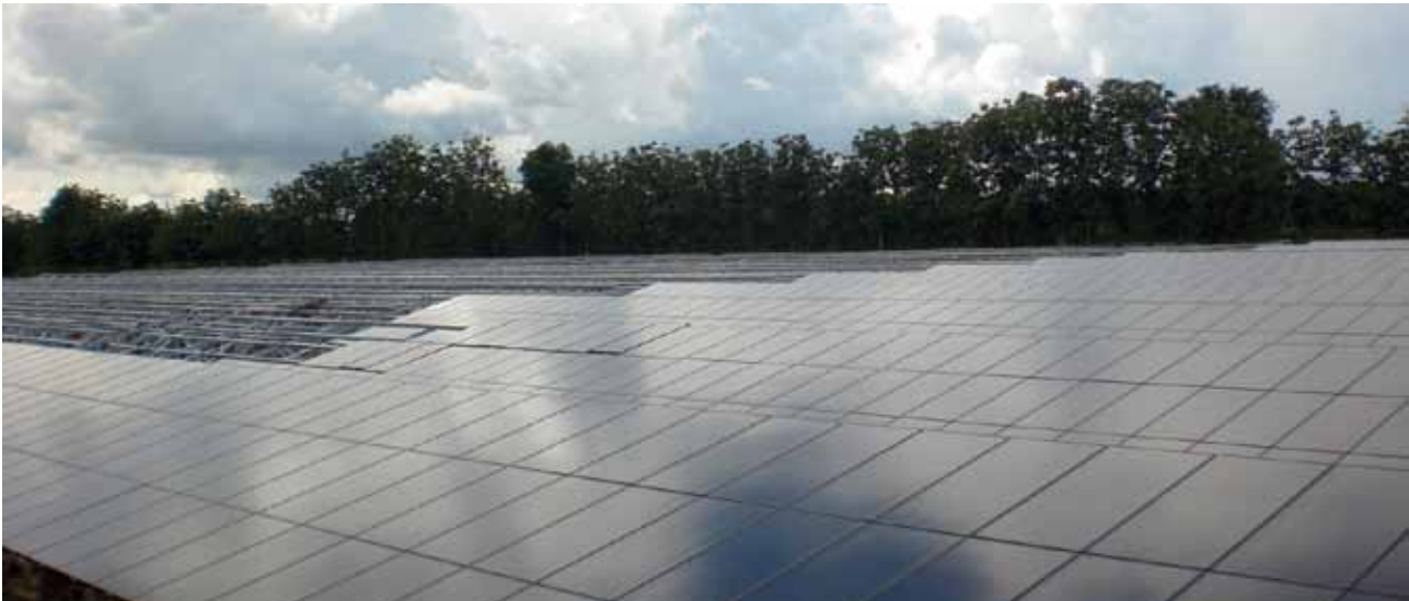
Gunkul's project will help the kingdom of Thailand reach its goal of installing 500 MW of solar power eight years ahead of schedule.
